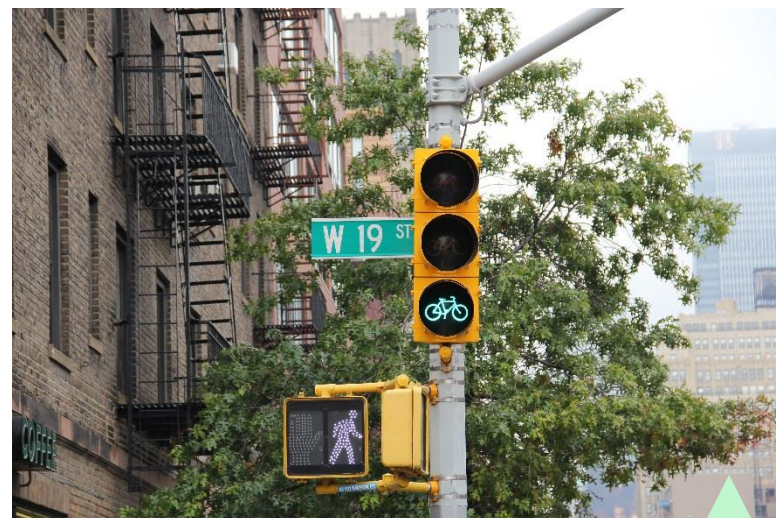
Bicycle signals are installed at Fully Split Phase Signal intersections
